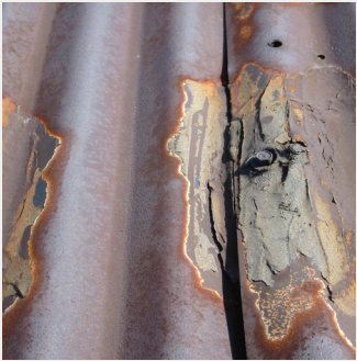
□ Rusted metal roof with fastener deterioration
