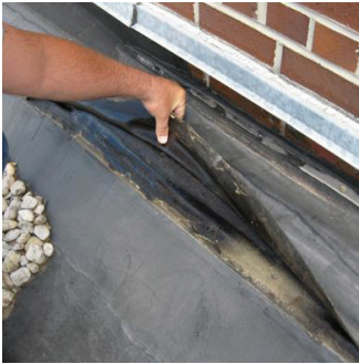
❑ Failed single-ply flashing
